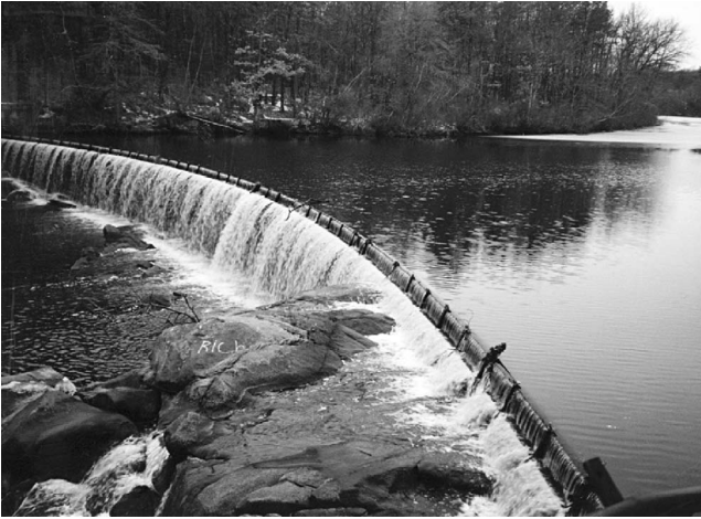
Fig. 3.7.8 Tupperware Dam on the Blackstone River (photo taken by Zhen-Gang Ji on February 3, 1998).
